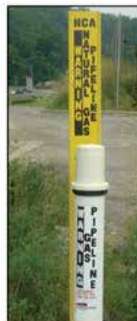
5. HCA marker and cathodic protection test station
